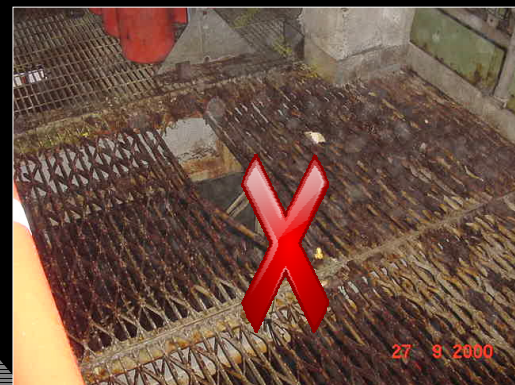
Corroded Steel Grating
