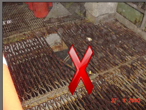
Corroded Steel Grating
